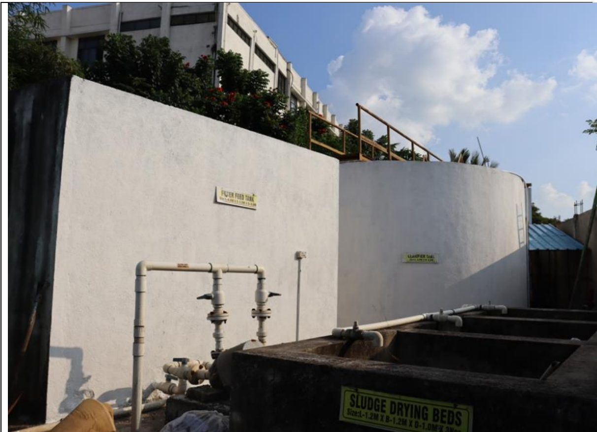
Filter Feed , Clarifier and Sludge drying Beds
