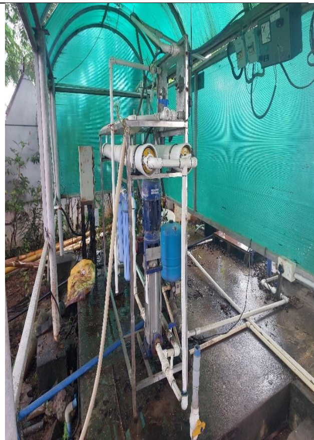
RO System Unit Covered By
