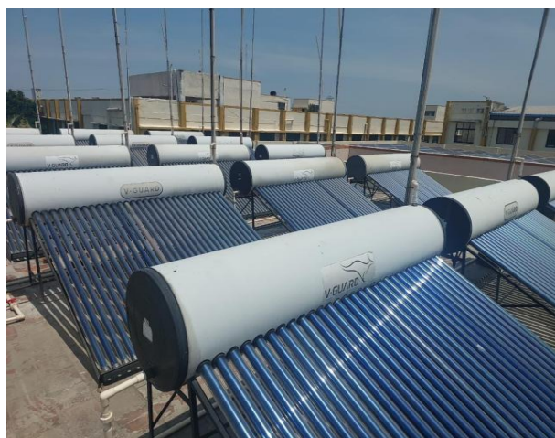
Solar Water Heater
