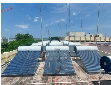
Solar Water Heater
