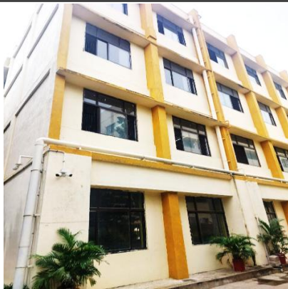
Rainwater Harvesting (Pipes)
