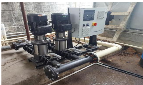
System provided with Adequate clearance
