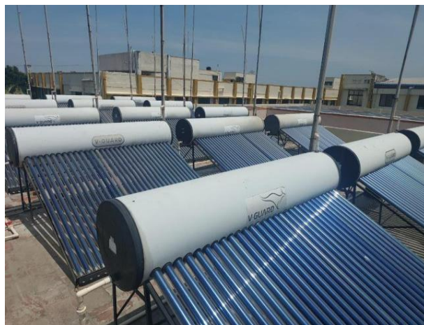
Solar Water Heater
